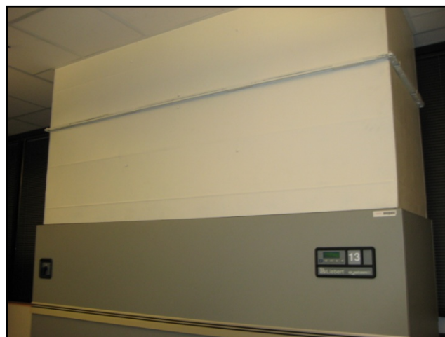
Figure 3: Ducting from ceiling plenum air return to opening of CRAH unit.
