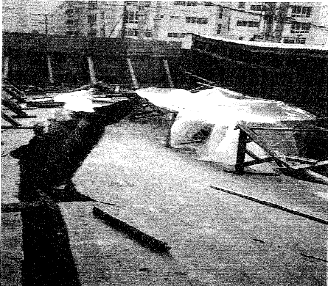
Figure 1. Active mode failure as seen from street level.
