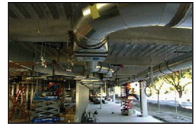
HVAC Duct installed exactly as shown in model
