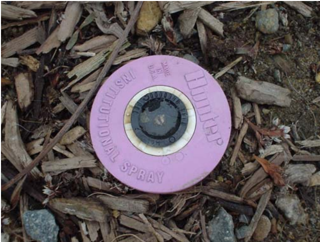
Fig. 10 – Purple-colored sprinkler head, indicating recycled water. This prevents guests and workers from mistaking it for potable water.
