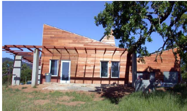
Figure 7: Stanford saved money using used redwood for the siding as opposed to new redwood.
