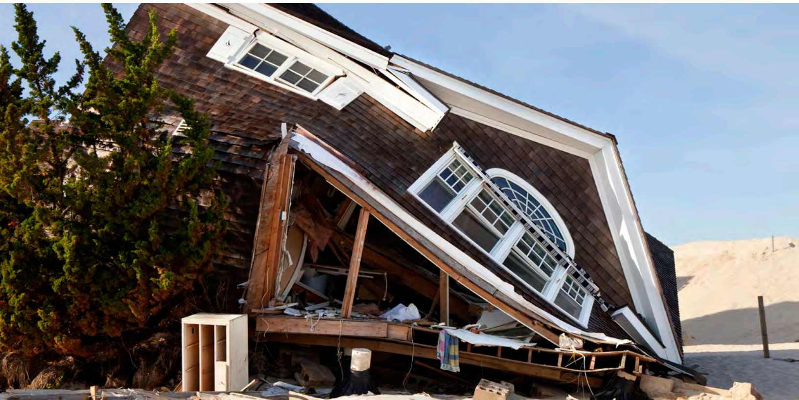
Damage caused by Superstorm Sandy. Courtesy of Thinkstock.com
