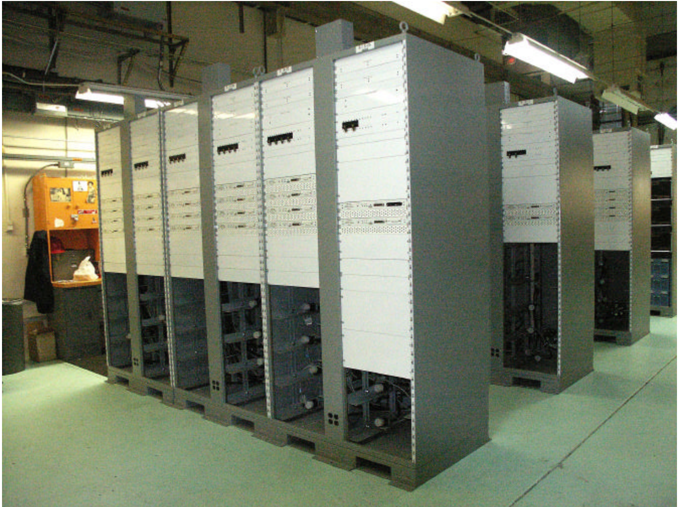
Intermediate Power Supply rack Line-up
