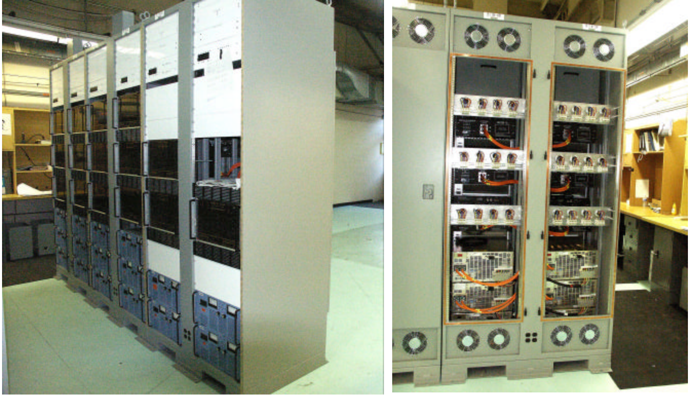
Bipolar Power Supply Racks – Front and Rear Views
