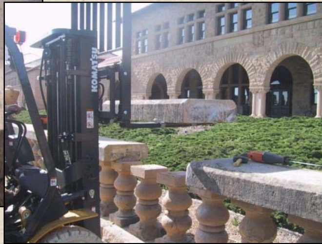
2. Top stones were removed. Mechanical keys existed between some top stones, making removal difficult in some cases.
