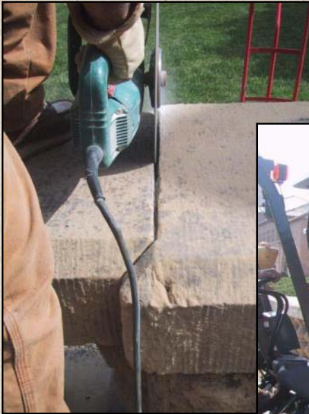
1. Joints between top stones were opened.
