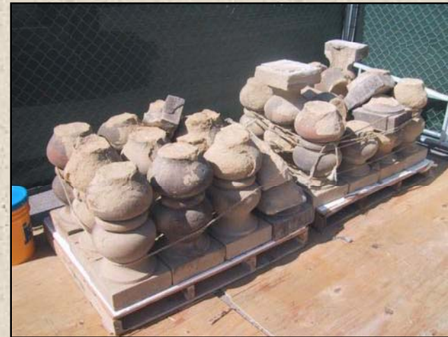
3. Balusters were first loosened (top) and then removed. Upon removal, the extent of decay became apparent, as the bottoms of nearly all the balusters fell off (bottom).
