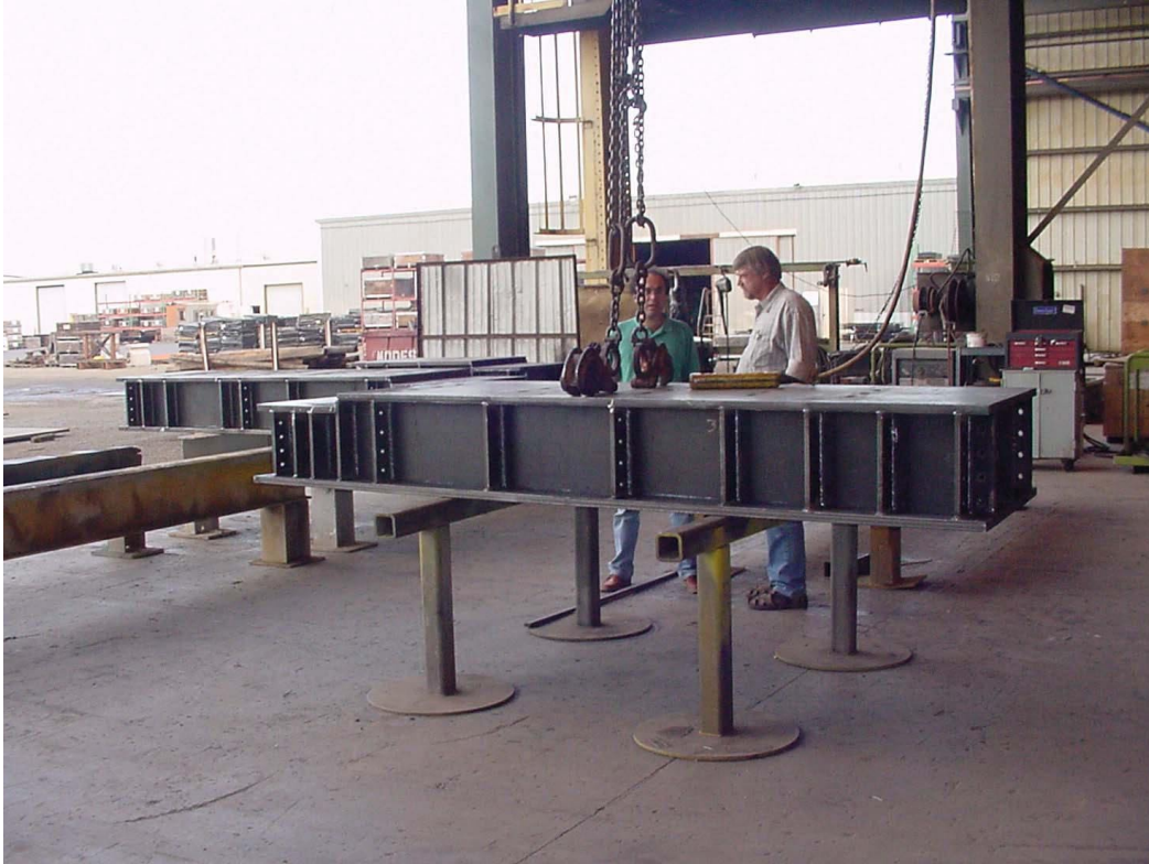
SSRL staff along side the 145D Type 1 Raft after completion in the welding sequence
