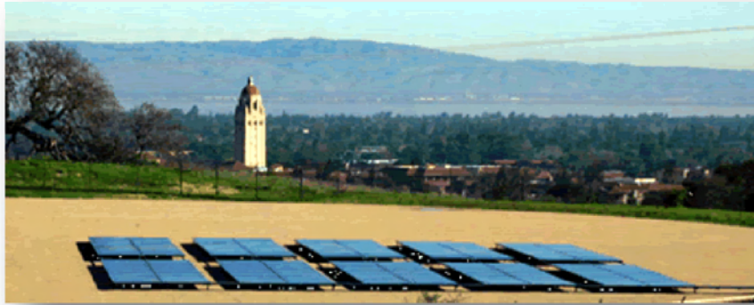
Photo: Photovoltaic Installation (powering the President's residence) on a Stanford water reservoir.
