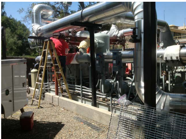
A new regional heat exchanger
