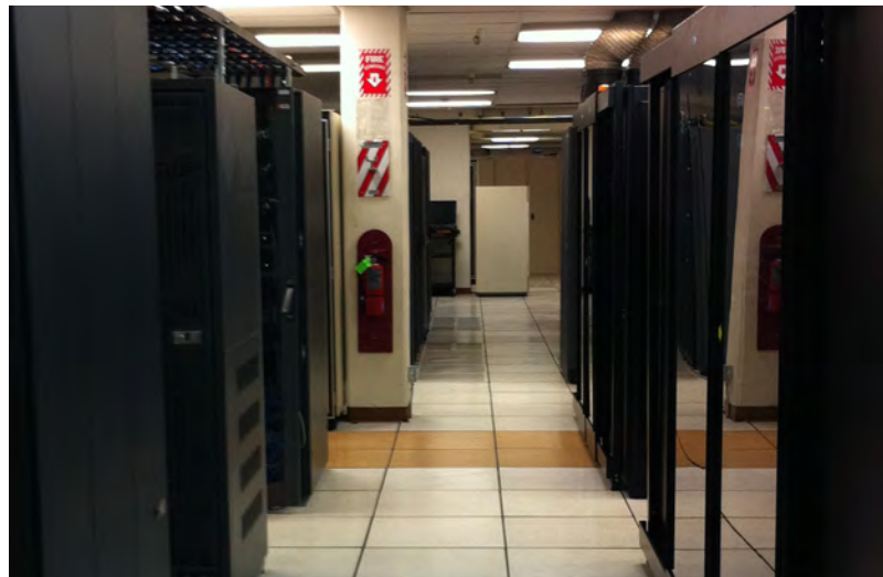
Photo: Data center end-aisle isolation
