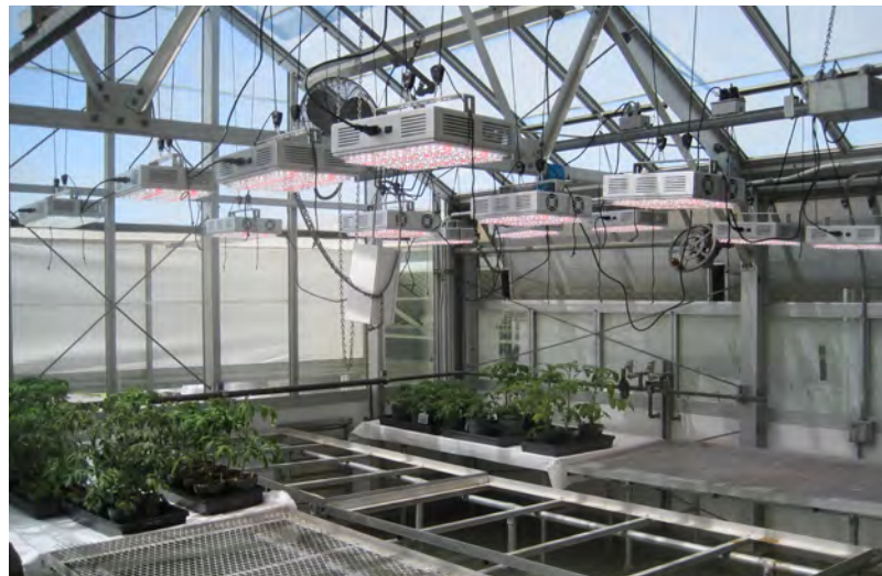
Photo: Department of Biology greenhouses were outfitted with efficient LED lighting under the ERP program, saving 248,000 kWh/year.
