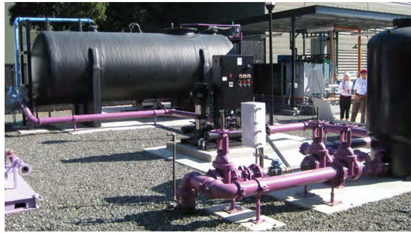
Photo: Stanford's recycled water facility supplies many new buildings, including the new Science and Engineering Quad and Knight Management Center.
