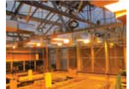
Greenhouse lighting prior to the retrofit.
