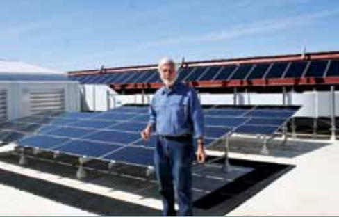
Professor Gil Masters stands in front of a solar photovoltaic installation on top of a Knight Management Center building.
