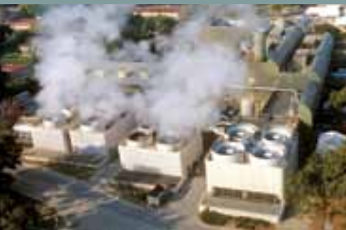
Cooling towers expel waste heat at Stanford's current Central Energy Facility.
