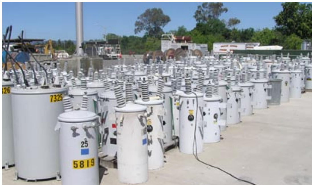
These Utility Department transformers are stored at the MSC—on a huge concrete pad designed and built specifically for that purpose
