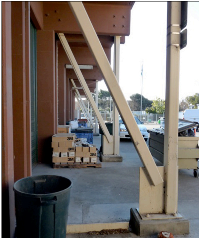
Figure 4-3. Despite external seismic bracing, the buildings at the Municipal Services Center are not expected to be usable after a major earthquake.
