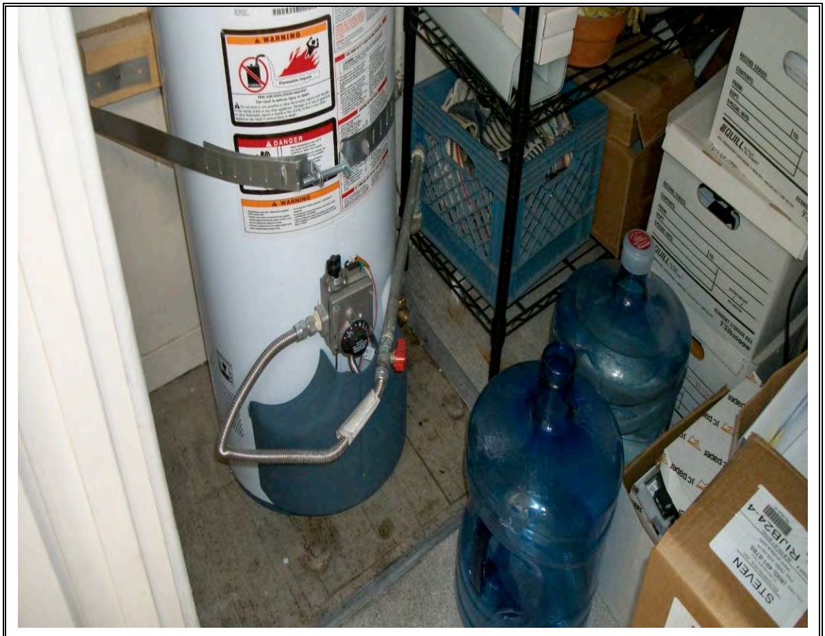
Photo No. 12: Water heater on the 2 nd floor of the building. Note the exposed wood floor.
