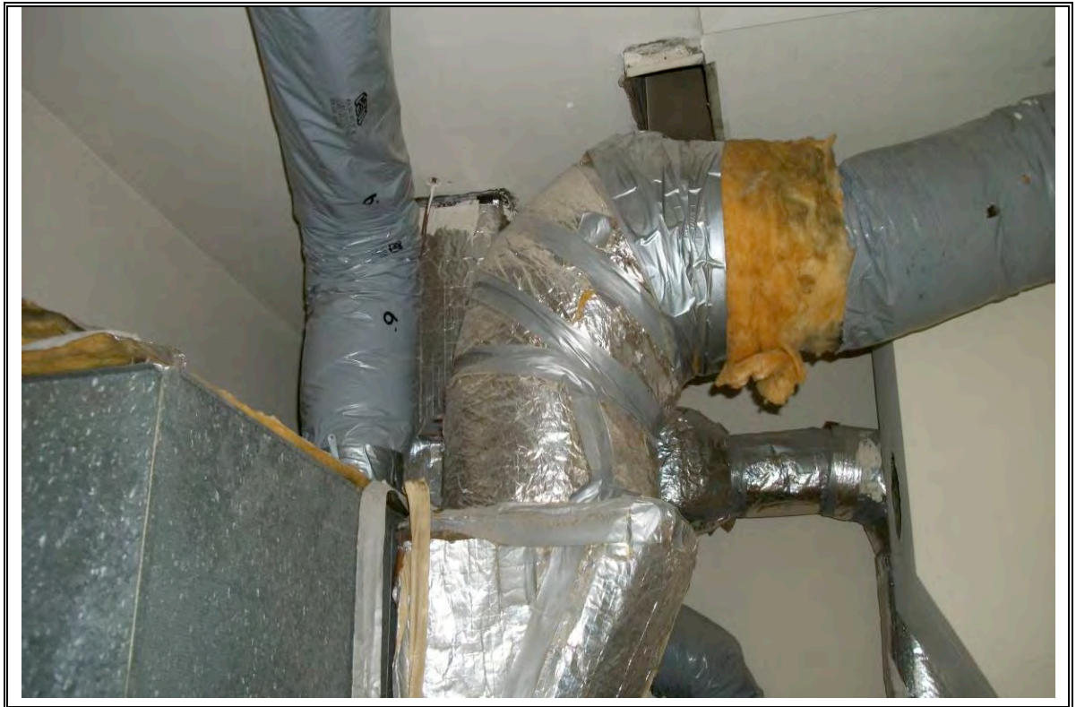
Photo No. 11: Fiberglass insulation and heater ductwork in a closet on the building 2 nd floor
