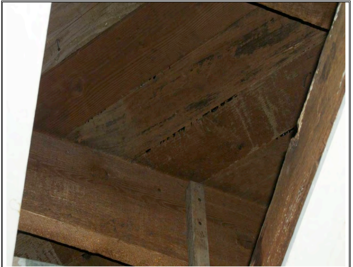
Photo No. 10: Looking up at interior framing of the building attic space
