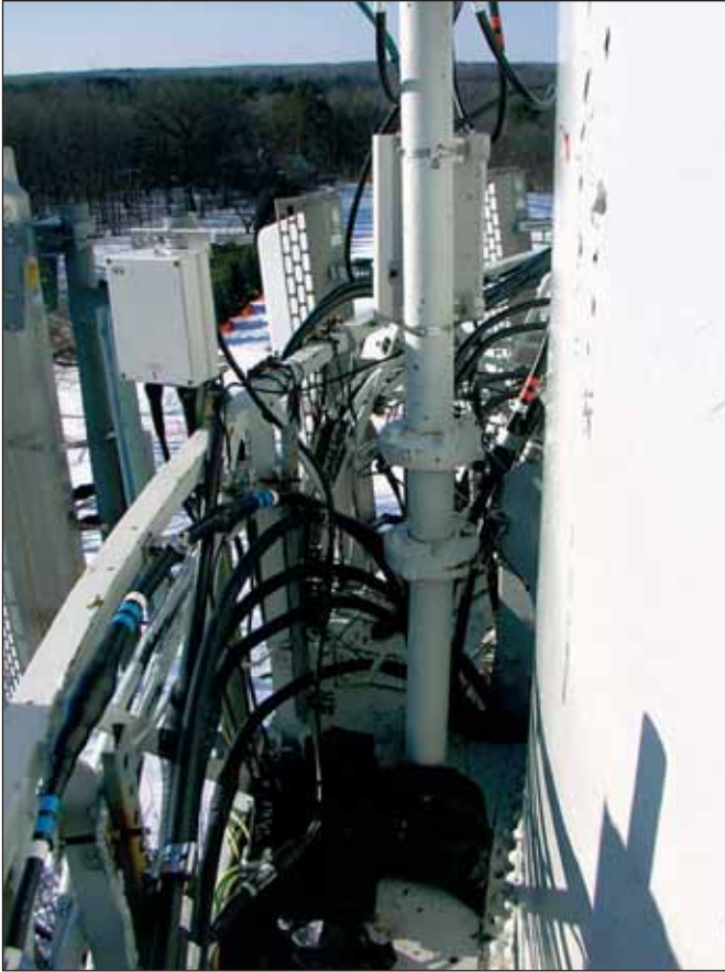
Figure 7.1 Crowded Cell Tower Installation
