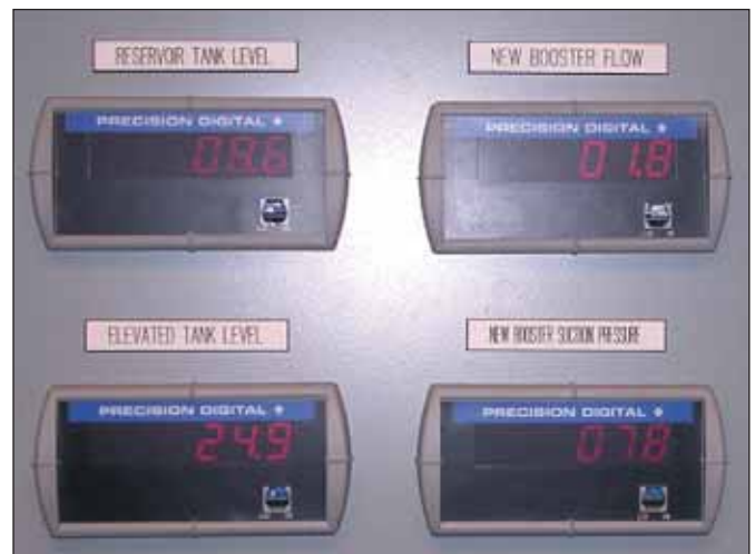
Figure 6.5 Readout meters for flow, water level and pressure from a SCADA system
