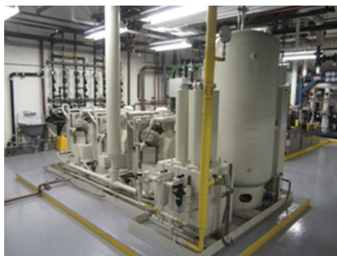
Medical air compressors
