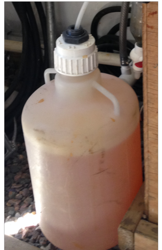
Figure 1: Ferric chloride feed reservoir
