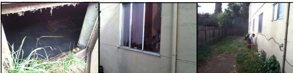
Left to right: stagnant water under a building in San Mateo; condensation on window; and Richard Chow using a backpack fogger to apply an adulticide treatment underneath the building.
