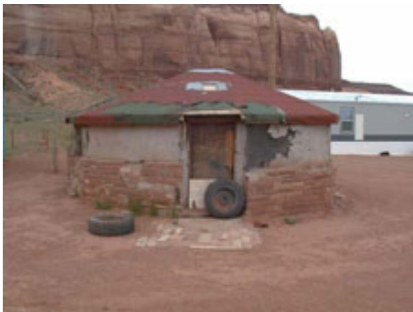
Hogan with Contaminated Foundation
