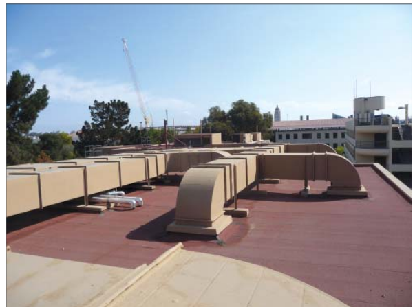
Forsythe Data Center - HVAC Renewal
