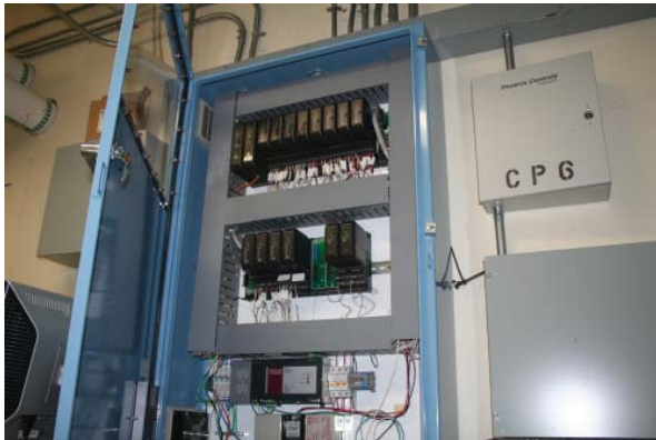
Stauffer 1 - Control Panels
