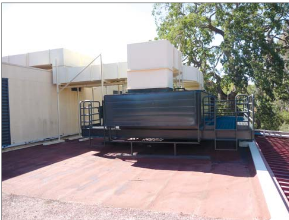
Forsythe Data Center - HVAC Renewal
