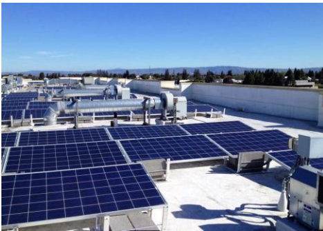
West-facing view of rooftop panels
