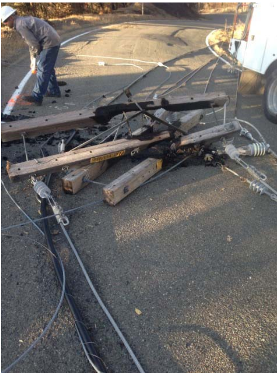
Palo Alto Utility Crews Clean Up Downed Power Poles and Help with Power Transmission Line Restoration
