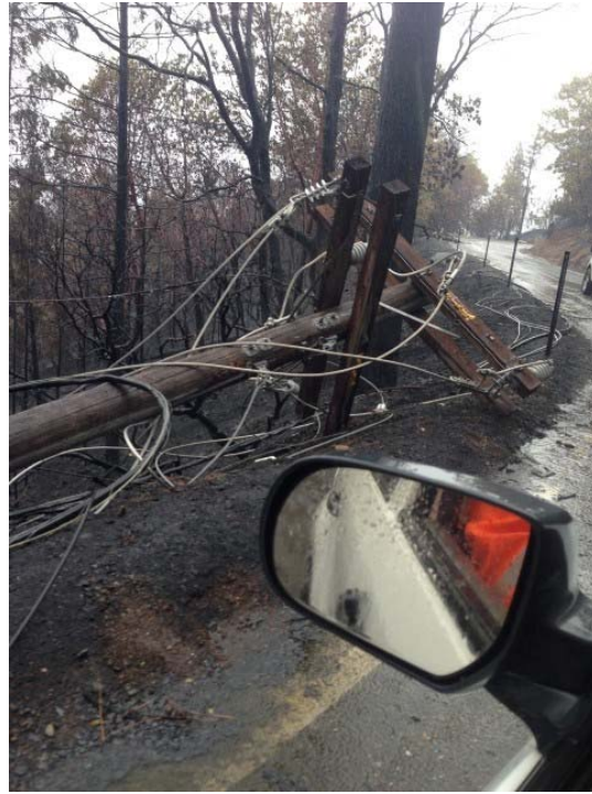
Power generating facilities, transmission and distribution equipment have been damaged.
