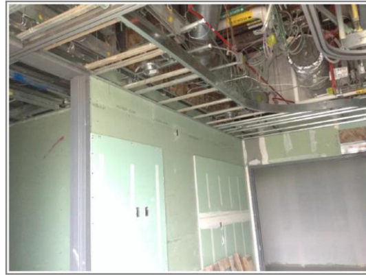
Room 3A111 ten weeks later on May 7, 2015. The drywall reveal panels were installed, about 2 hours' worth of work.
