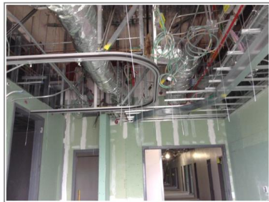
Room 3A131 ten weeks later on May 7, 2015. Sheetrock was added on the right wall and the stub wall near the door, about 2 hours' worth of work.
