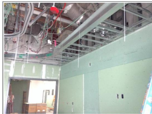
Room 3A171 ten weeks later on May 7, 2015. The drywall reveal panels were installed, about 2 hours' worth of work.
