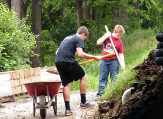
Community organizations, school groups, and volunteers helped build and design elements of Riverfront Park. Eagle Scouts built a retaining wall to help mitigate flooding.
