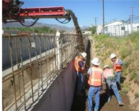
Figure 35 What is this crew doing? They are located on the East-end, on the North sub-location, they are the earthwork discipline, engaged in the backfill activity, with aggregates resource, for structural backfill, narrow fill operation, conveyor method, internal laborers crew on regular time, and internal material and equipment; haul type is not visible. The CIFE-AROW 187 activity name for this operation: place ¾" aggregate trench-wall structural backfill, east-end north.
