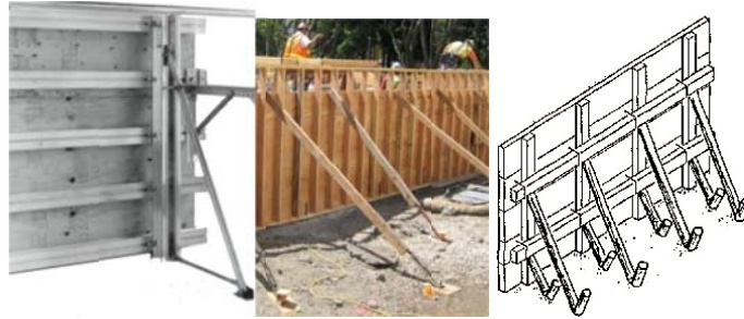
Figure 68 Three visions of formwork; as laborers we had not seen formwork higher than a 10" highway cross section and did not have reference material. The superintendent saw the design on the left (carpenter panels). Based on 'Vitruvi' experience we framed and sheeted forms similar to those in the middle (like a house wall). A journeyman mason saw the design on the right (mason forms).
