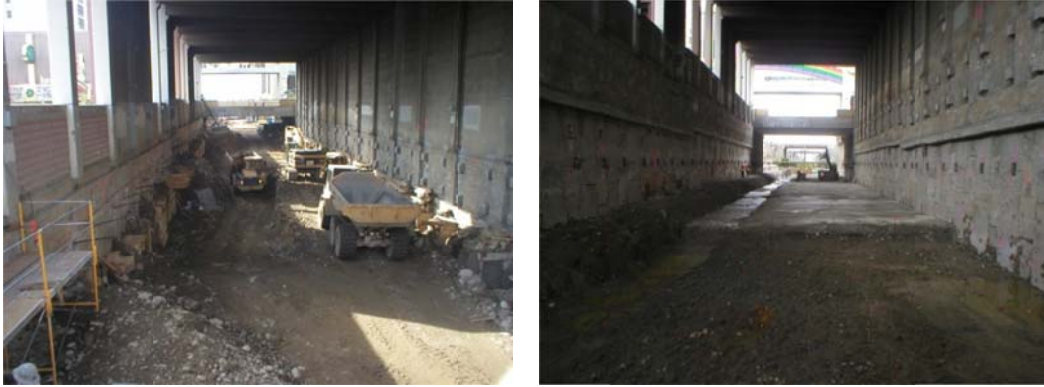
Figure 42 Example operation the earthwork field engineer measured as a visual percent complete. The image on the left is the current state and the image on the right is the finished state, what is the current percent complete, 5%?
