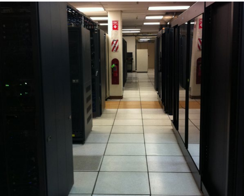
Photo: Data center end-aisle isolation
