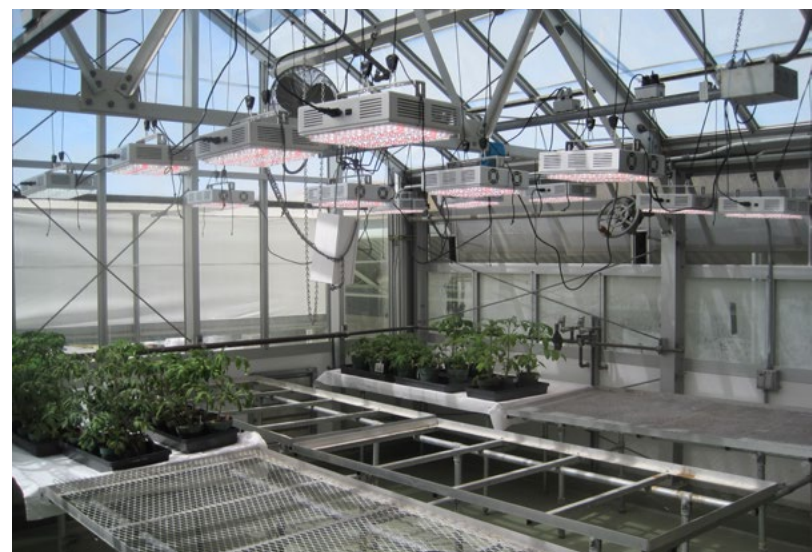
Photo: Department of Biology greenhouses were outfitted with efficient LED lighting under the ERP program, saving 248,000 kWh/year
