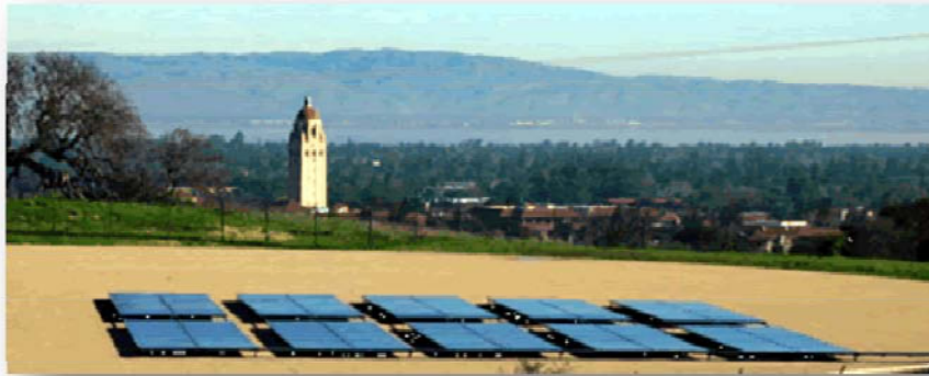
Photo: Photovoltaic Installation (powering the President's residence) on a Stanford water reservoir.
