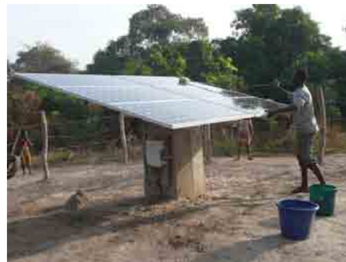
The completed solar panel will now provide power to irrigate crops.
