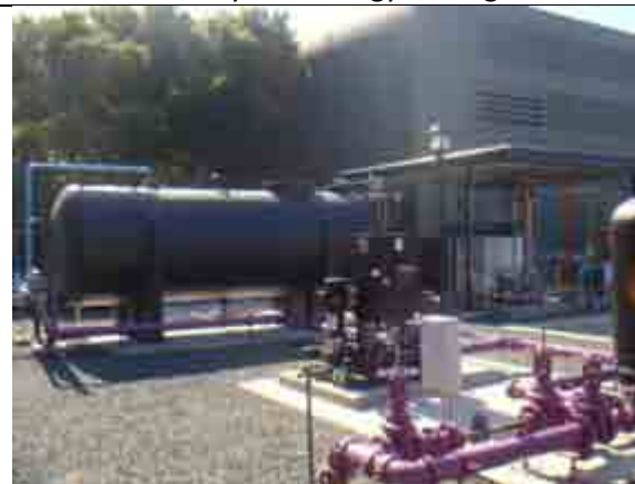
Reclaimed water plant located inside Central Energy Facility
