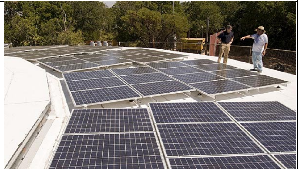
Stanford energy engineer Scott Gould, left, talks with Greg Gillette of REC Solar amid the 252 polycrystalline panels mounted on a partially buried water tank (known as the San Juan Reservoir) near Hoover House. The multiple levels of the historic dwelling made placing the panels on top impractical.
