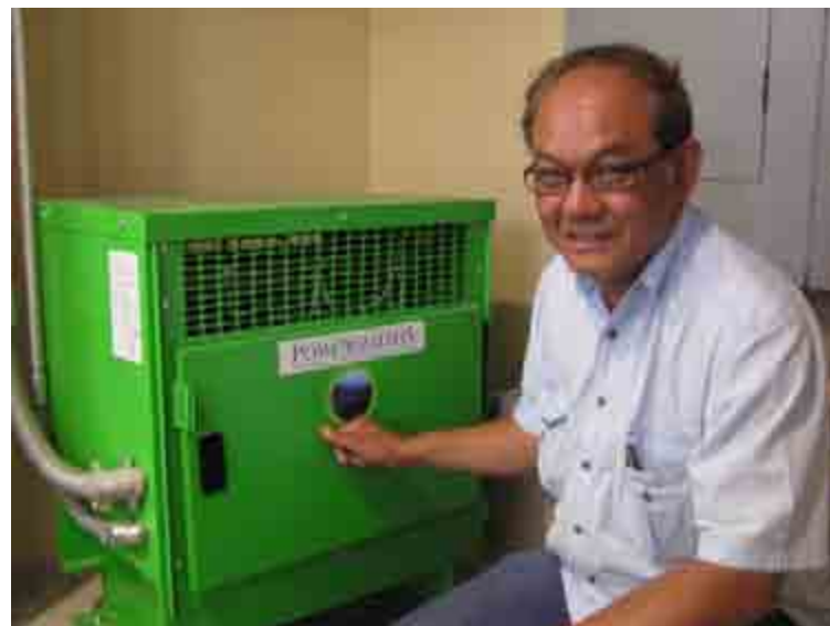
Tai Tran, Zone C Engineer, next to the high efficiency transformer provided by Powersmiths
