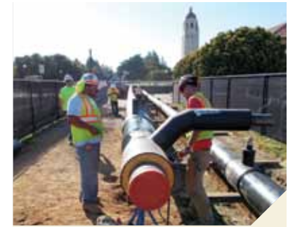
DPM is managing design and construction for 20 miles of underground hot-water pipe installation for SESI – half of which has already been completed.
