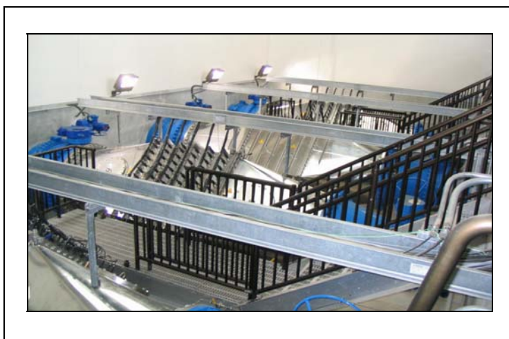
Figure F.13. UV Reactors at the Weber WTP No. 3 (3 duty + 1 standby reactor in parallel)
