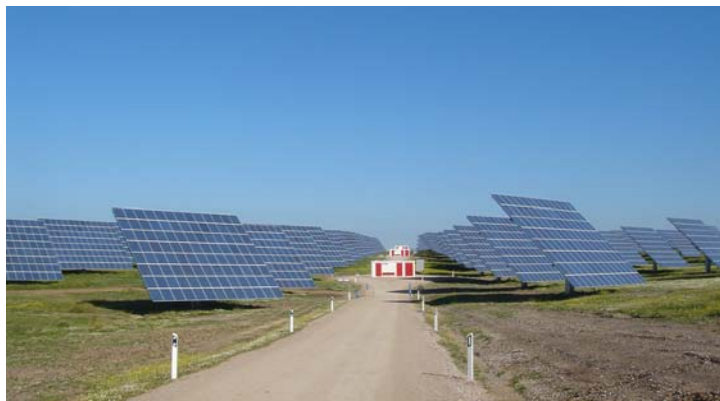
27 28 Figure 3.12: A portion of the 42-MW grid-connected PV power plant in Moura, Portugal.
