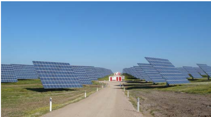
Figure 3.12: A portion of the 42-MW grid-connected PV power plant in Moura, Portugal.
