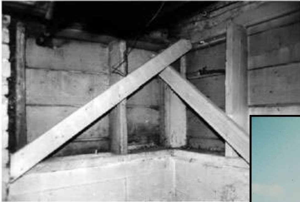
Figure 16. Shows an inadequate pony wall bracing that does not meet the requirements. (Photo by Gary Milici, RetroFitters Inc.)
