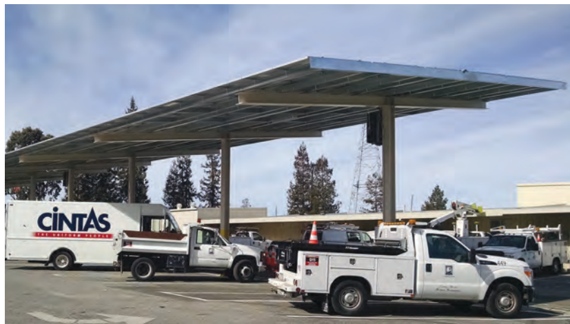
The City's Service Center now enjoys the benefits of newly-installed solar panels.
