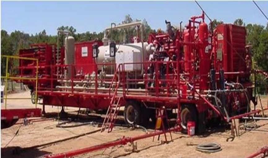
Green Completion Equipment (source: Weatherford)
