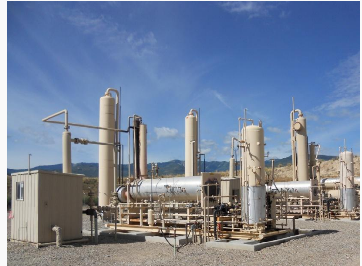
Well Production Pad with Glycol Dehydrators (tall columns) (source: EPA)
