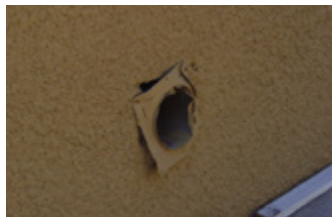
ProBest seals holes such as this one found at Precious Treasures with caulking and either steel or copper wool to prevent pest access.
