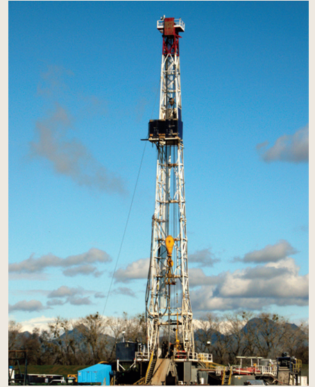
A gas well in central California with the Sutter Buttes in the distance.
