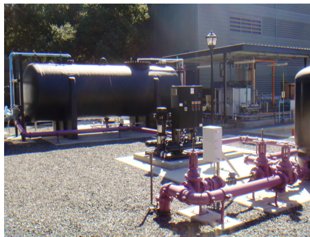
CEF Recycled Water Plant
