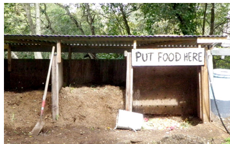
Water catchment system installed at Synergy's compost site
