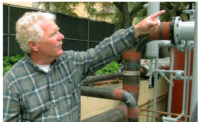
Dean Murray, Associate Director, Thermal Energy Distribution, explains the heat exchange station
