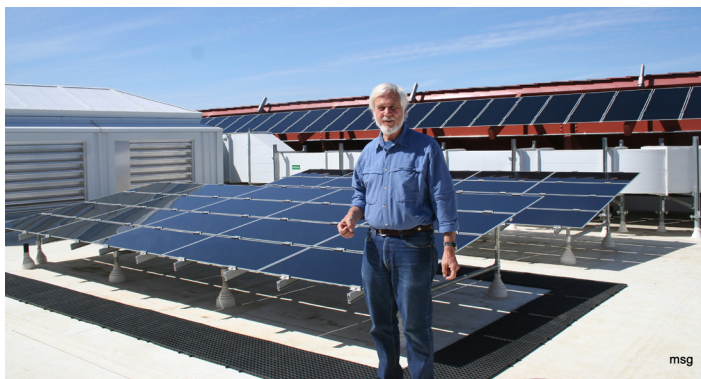
Gil Masters stands near a PV array on the KMC roof. Photo credit: Scott Gould
