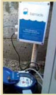
The barnacle water meter provides real-time monitoring to help identify water leaks at specific campus locations.
