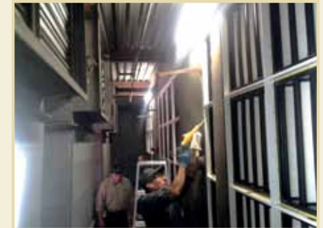
Members of Stanford's HVAC shop installed improved filtration media that saved more than $26,000 annually at the Clark Center as part of the Energy Retrofit Program.
