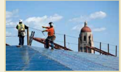
The final building in the new Science and Engineering Quad, to house Bioengineering and Chemical Engineering, is currently under construction.
