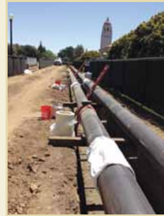
Work to convert the campus from steam to hot-water systems has already begun and is being carefully timed to minimize disruption to the campus community.
