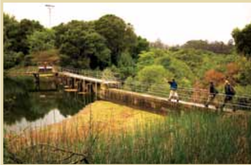
Searsville Dam and Reservoir, built in 1892 and owned by the university, is the subject of a multiple-year study.
