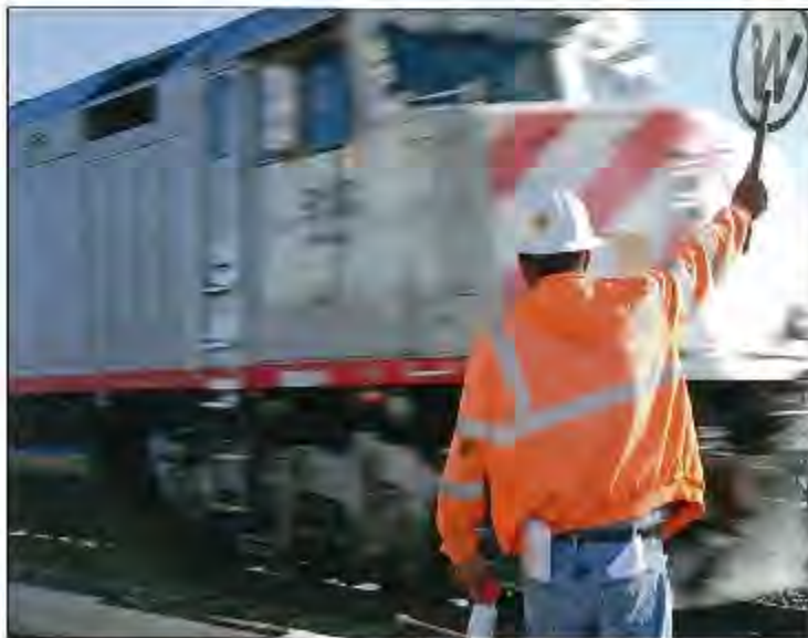
Spotlight is on the Watchman who keeps everyone working on the right of way at the San Bruno Grade Separation Project and other Caltrain rail projects safe and alert to trains on the tracks.
