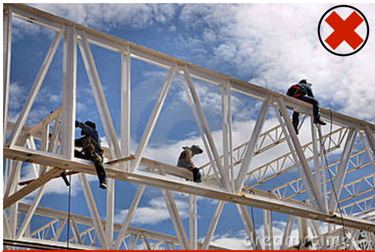
High potential fall hazard
