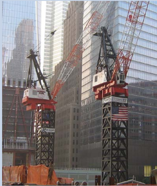
Two Cornell Tower Gantry Cranes operating in Lower Manhattan at the site of Three World Trade Center.
