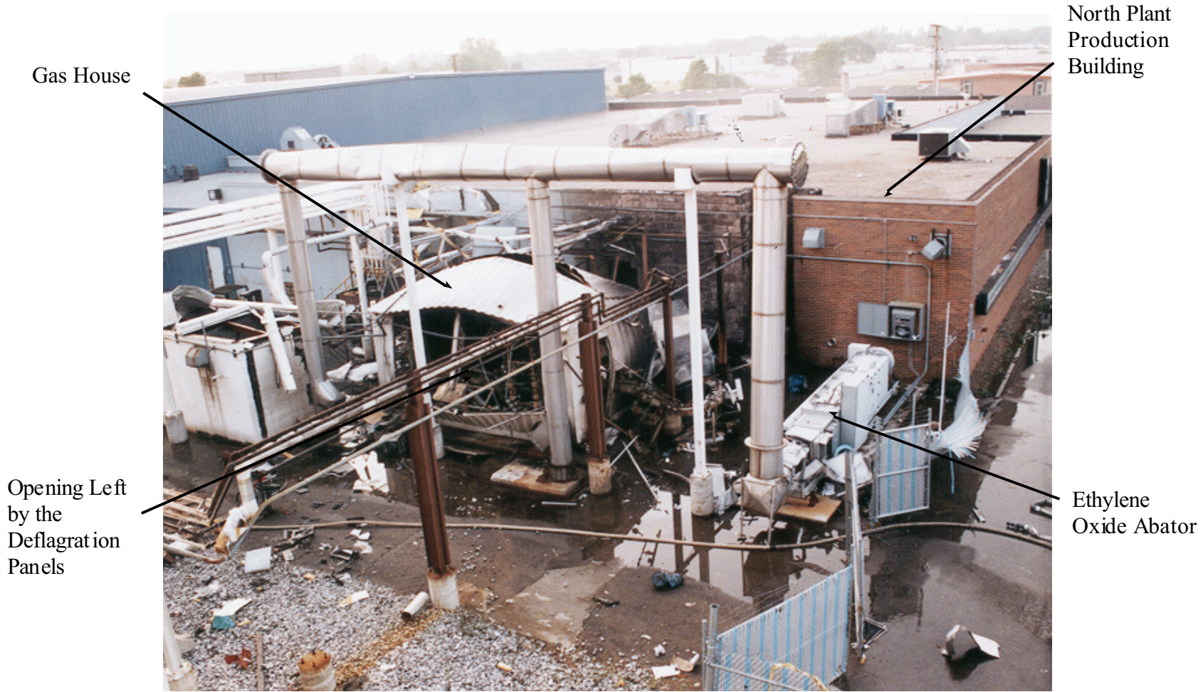
A-1: The Gas House and the Production Building after the explosion and fire.
