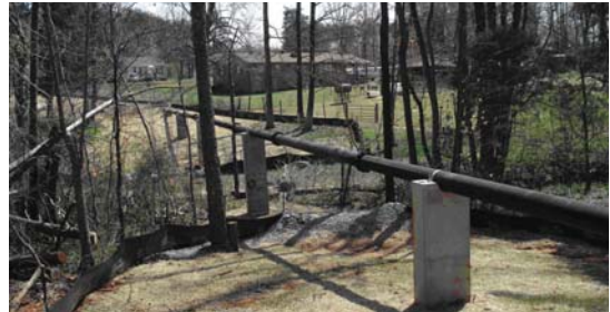
First-time sewer installation for 51 homes in West End Community stops septic tanks from overflowing and creating a stream of sewage that threaten drinking water. Project was funded by a million dollar block grant and City of Mebane matching funds in 2008.
