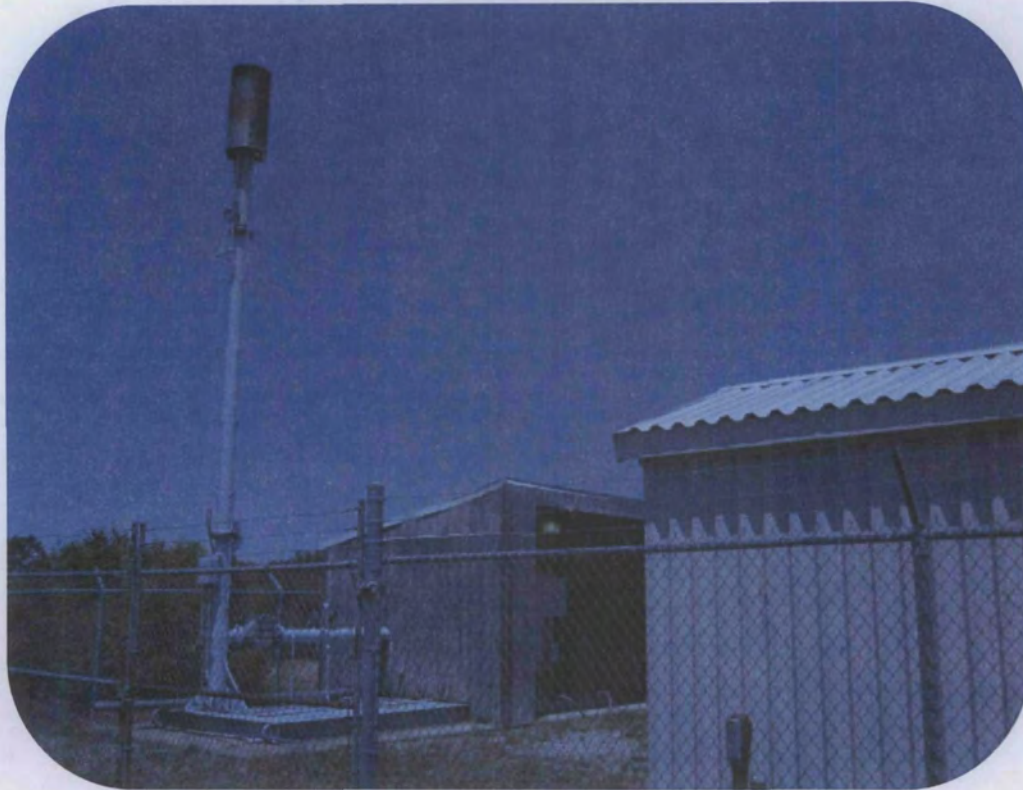
Photo 15: On site, landfill gas candlestick flare, landfill gas system structure, and associated storage structure.
