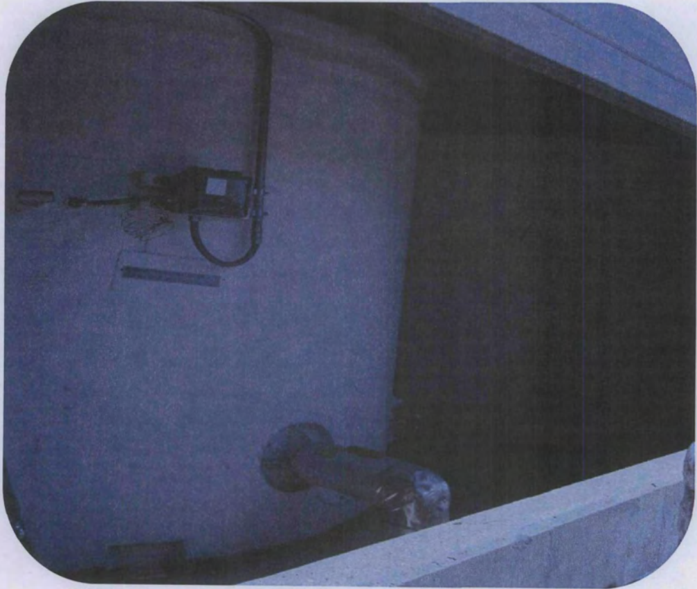
Photo 17: Condensate storage tanks contained within structure on site.
