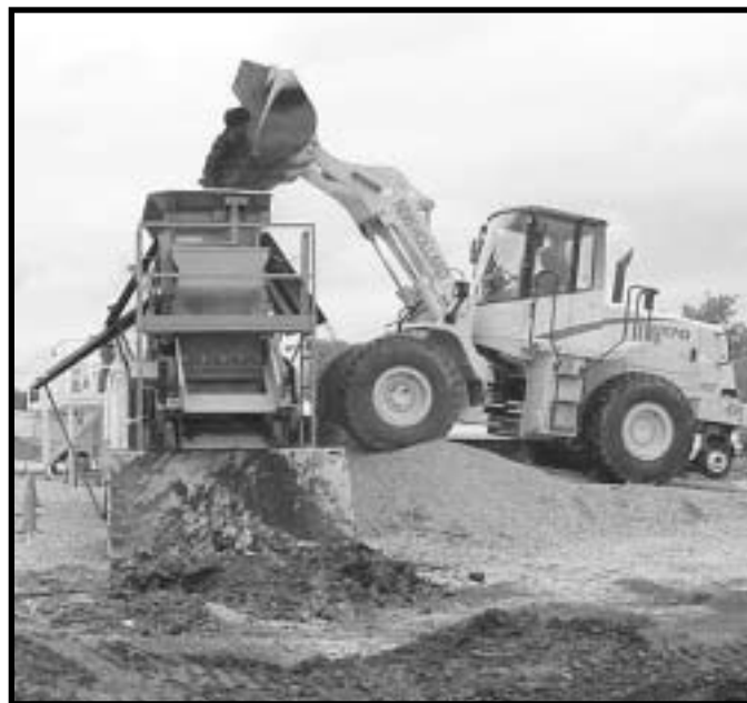
The segmented gate system is loaded with soil from NPL-8. The system detects contamination and sorts the soil per cleanup standards.
