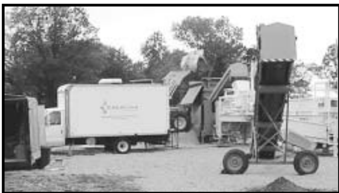
Equipment for the segmented gate system is set-up on-site.
